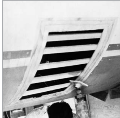
Figure 5-16 Bevel the edges and fasten temporary stringers to the back of the opening.
