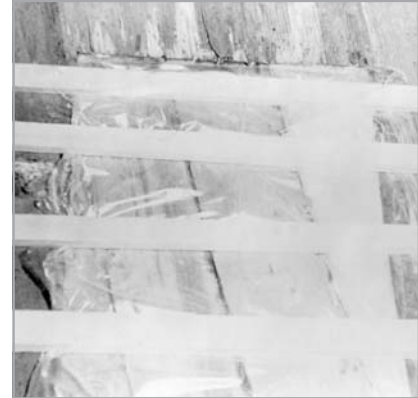
Figure 5-17 Cover the stringers with plastic to prevent bonding. (View from inside of hull).
